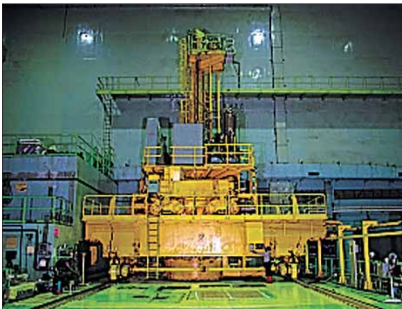
Fuelling machine of DHRUVA, which loads and discharges nuclear fuel
