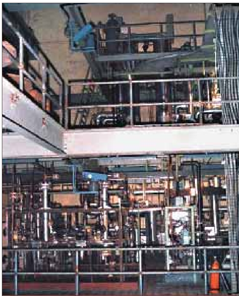
3 MW boiling water loop
