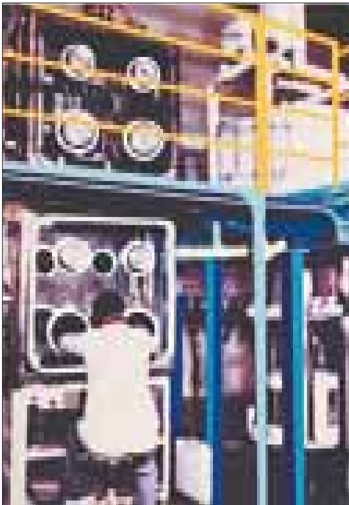
View of fuel handling facility of PURNIMA-2
