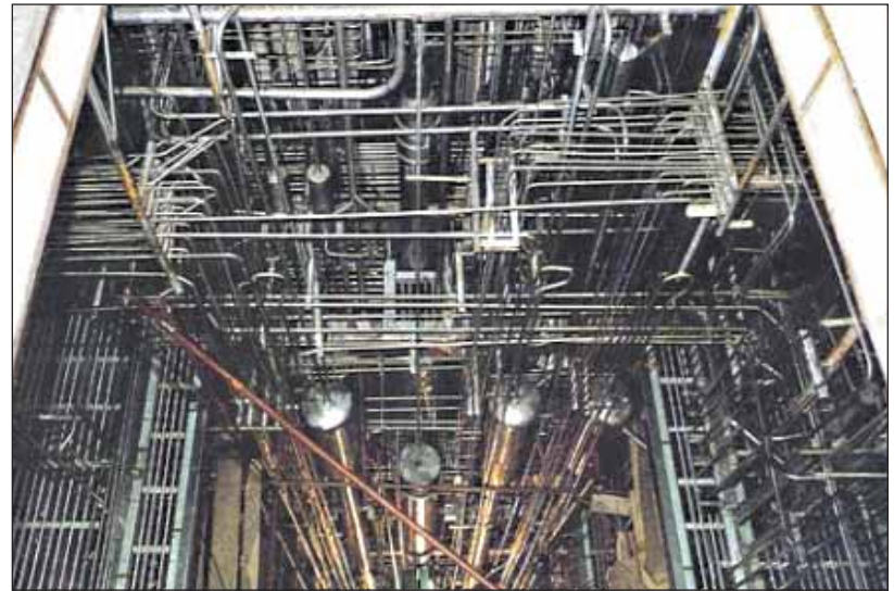
Typical cell piping in reprocessing plant
