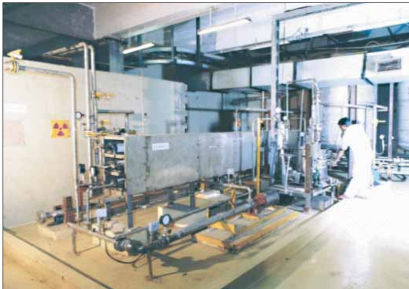
Reverse osmosis plant at waste immobilisation plant, Trombay
