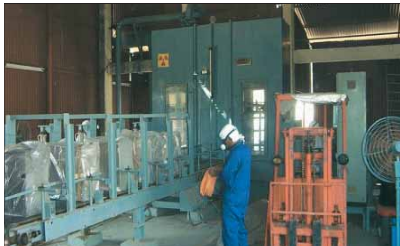
Compaction unit for radioactive waste drums and HEPA filters
