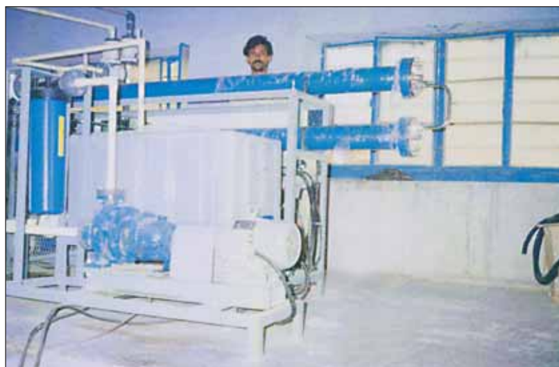
Reverse osmosis plant at Saltana village, Jodhpur, Rajasthan
