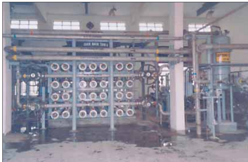
Sea Water Reverse Osmosis (SWRO) plant building and membrane modules at Kalpakkam (Top and Bottom)
