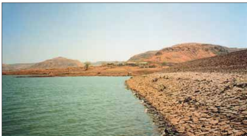
A view of the Chaskaman dam in Maharashtra where radiotracer experiments provided information about the seepage sites
