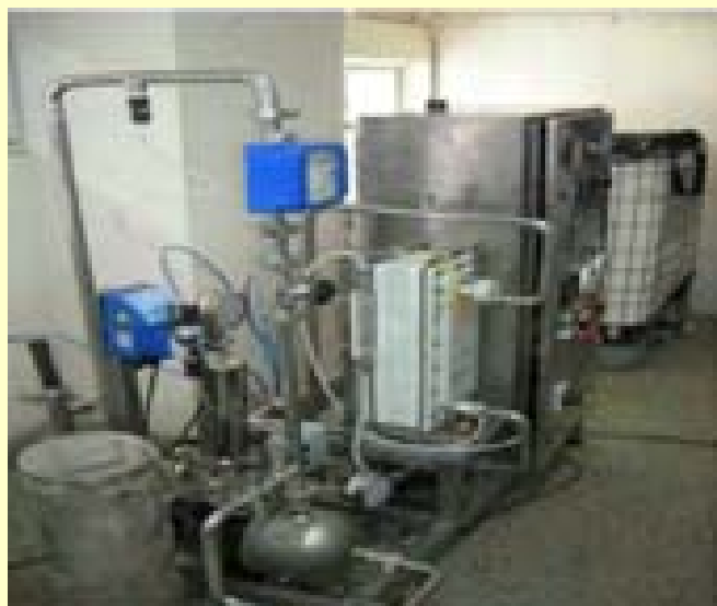
Electro-De-Ionisation unit (capacity: 5000 litres/day)
