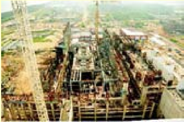
Overall view of Power Island
