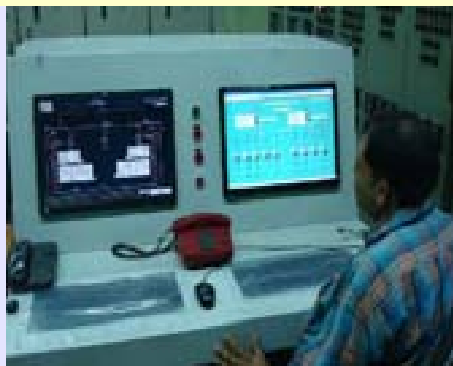
SCADA control panel of new MA set
