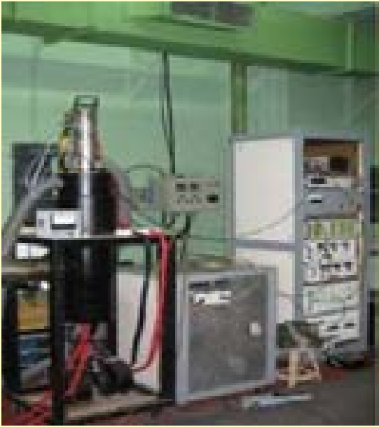
14 kW @ 350 MHz RF system
