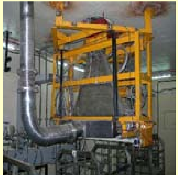
10 MeV RF Linac System on the ground floor
