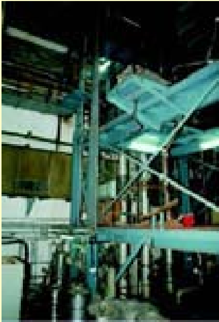
Modified Heavy water upgrading plant
