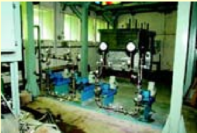
Electrolytic Cell of Combined Electrolysis Catalytic Exchange unit
