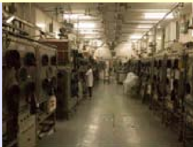
New fabrication line of Advanced Fuel Fabrication Facility for PFBR (BARC)
