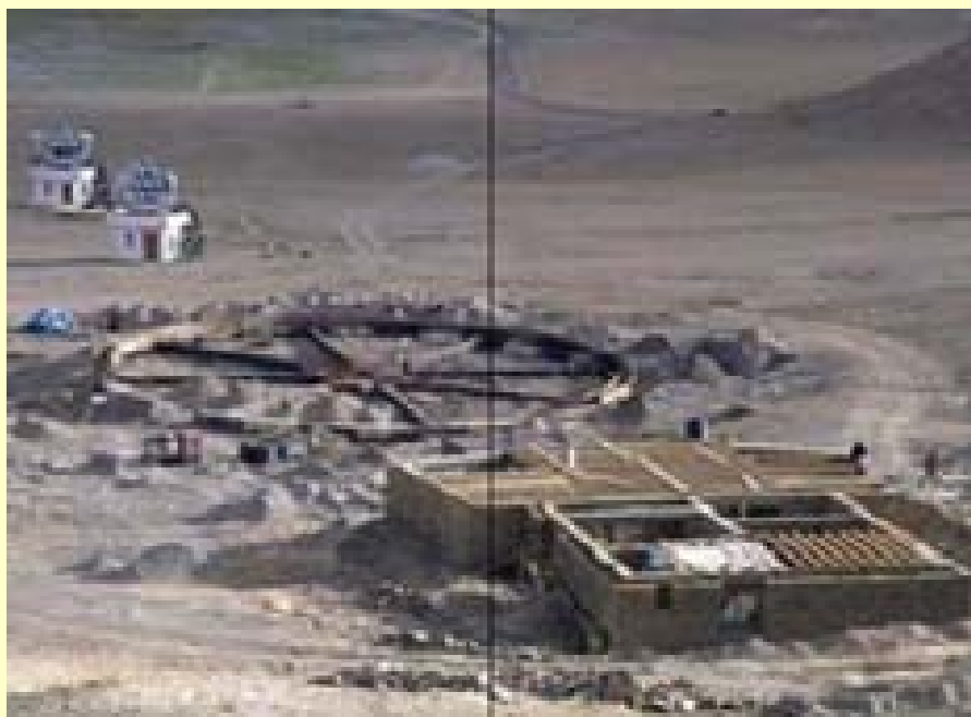
21 metre Major Atmospheric Cerenkov Events (MACE) Telescope under construction for Gamma Ray Hanle Astronomy in Ladakh (photo:ECIL)
