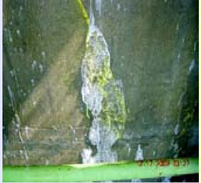
First Appearance of Crack at MAL with Soap Bubble Test in BARCOM Test Model during Over-Pressure Test
