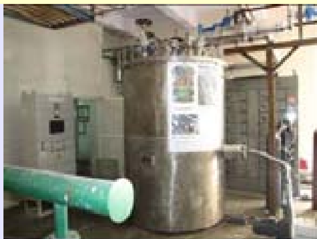
Helium Liquefier cold box connected to HP and LP lines of process compressor
