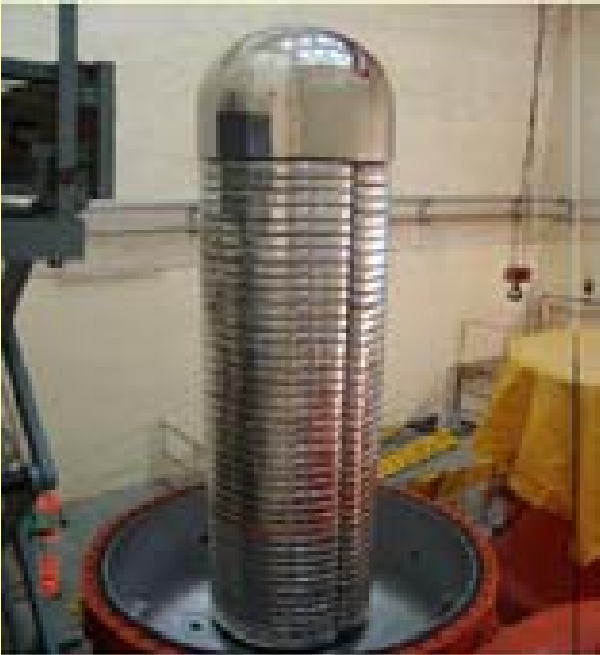
High Voltage Multiplier Column on the first floor
