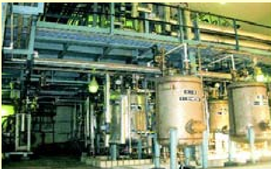
Boron Exchange Distillation Plant at Heavy Water Plant, Talcher
