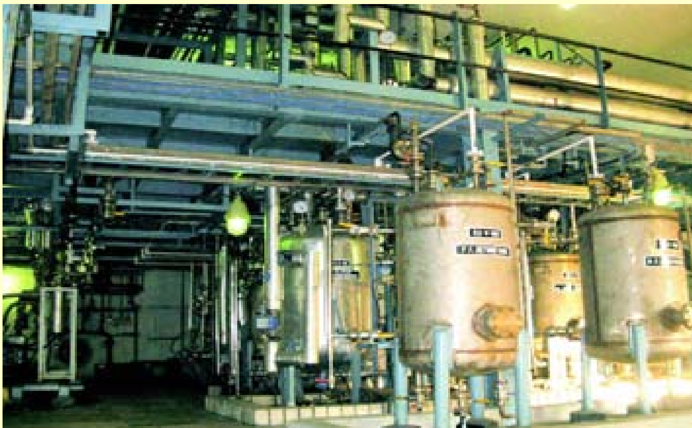
Boron Exchange Distillation Plant at Heavy Water Plant, Talcher
