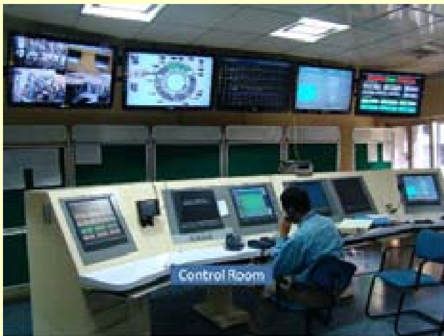
Control room of Superconducting Cyclotron
