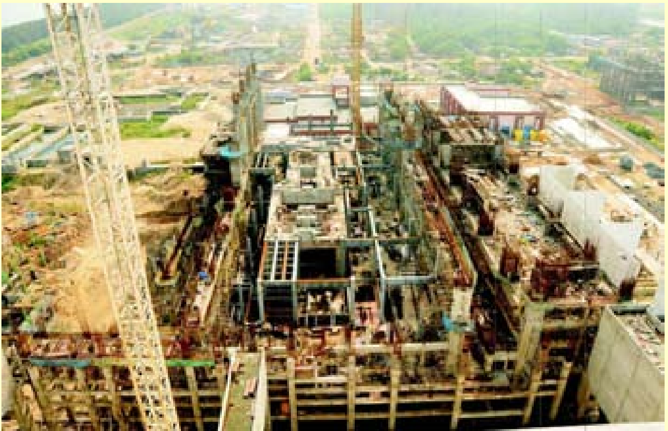
PFBR Project : Overall view of Power Island
