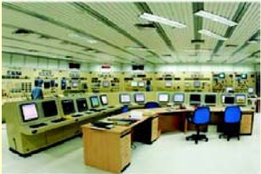
A modern Control Room built by ECIL for PHWR
