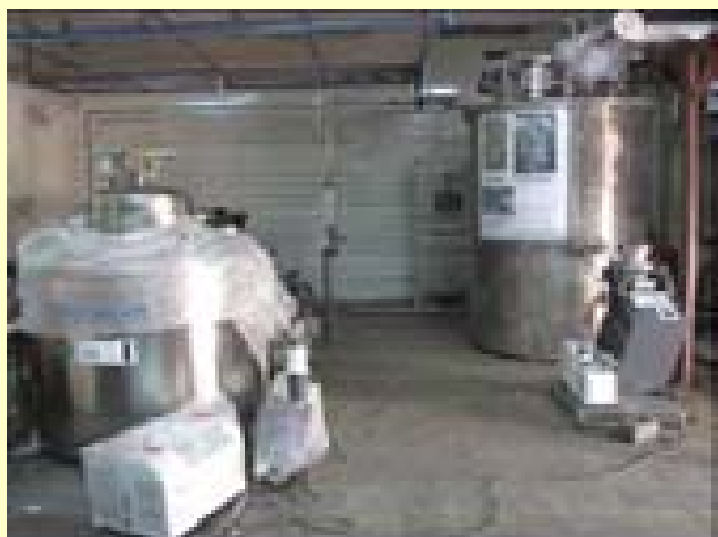
Helium liquefier cold box being integrated with process compressor and Dewar
