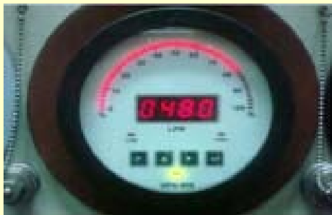
New Electronic Differential Pressure Indicating Switches (EDPIS) gauge of Dhruva
