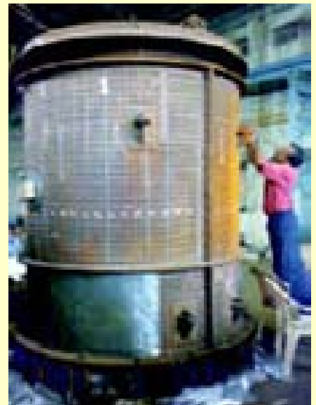
Lead shielding for sodium condenser arrangement
