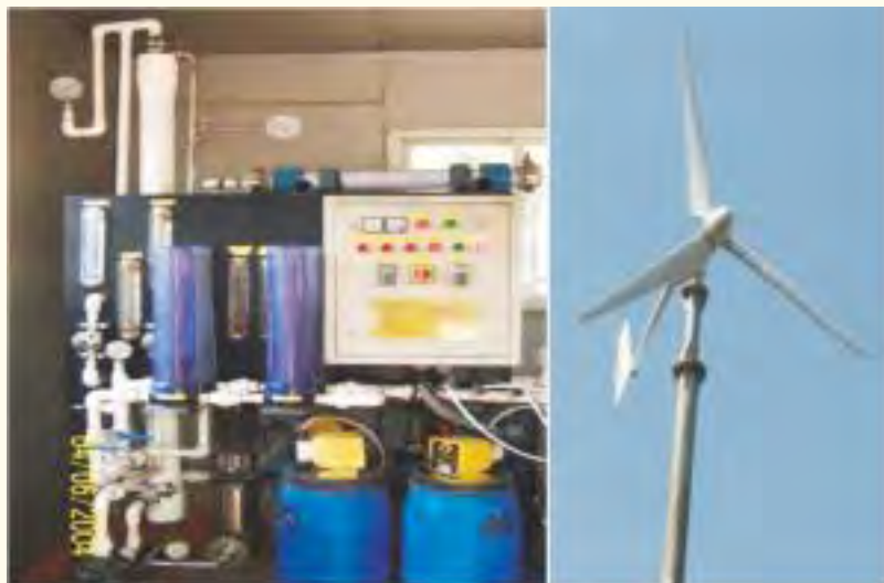
Brackish Water Reverse Osmosis Unit powered by wind energy at Trombay
