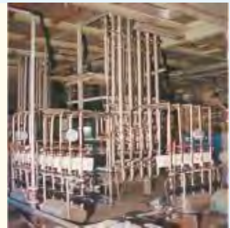
Tail pipes with Instrumentation
