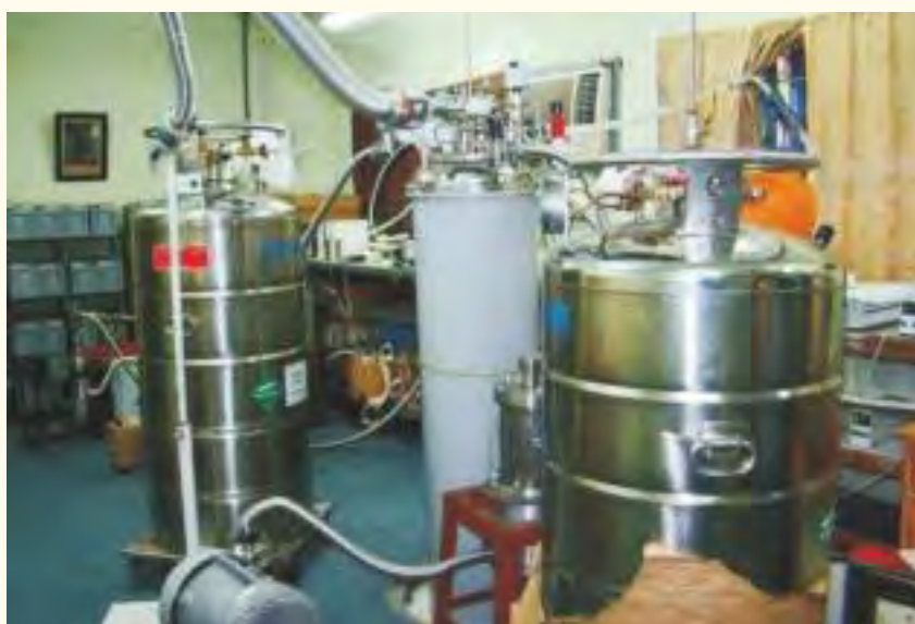
Helium Evaporator in operation
