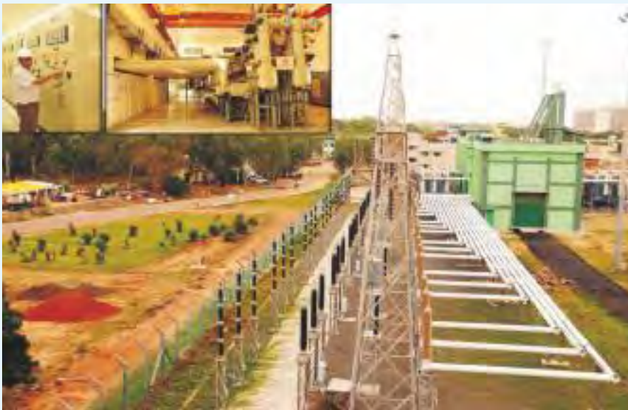
Switchyard commissioned by BHAVINI
