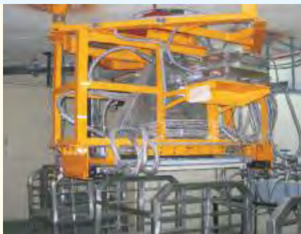
RF Linac assembly at EBC First + Ground Floor View
