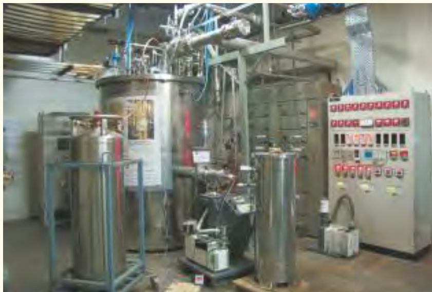
Helium liquefier under commissioning
