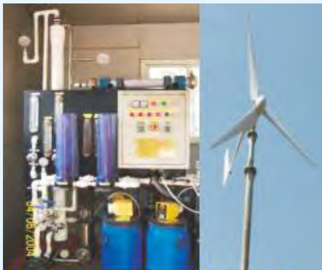
Brackish Water Reverse Osmosis unit at Trombay. This unit is powered by wind energy
