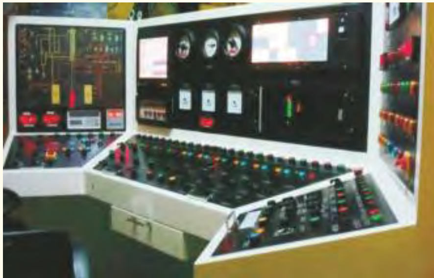
Renovated Fuelling Machine control panel
