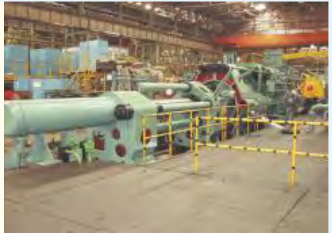
Extrusion press after revamping
