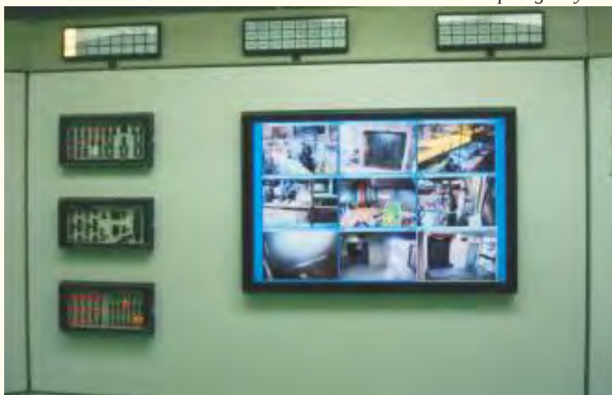
Refurbished Panel-C of control room
