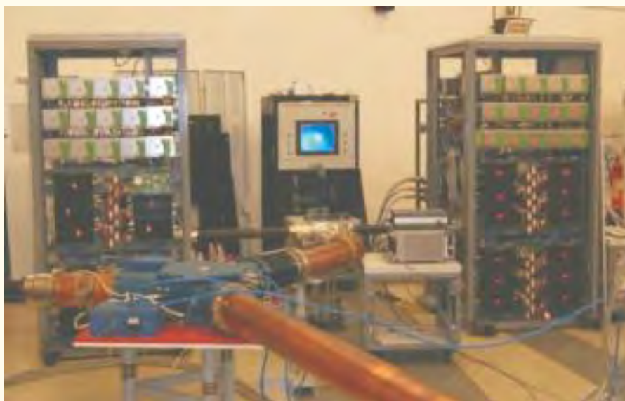
Two units of solid state RF amplifiers coupled to RF station-1 of Indus-2
