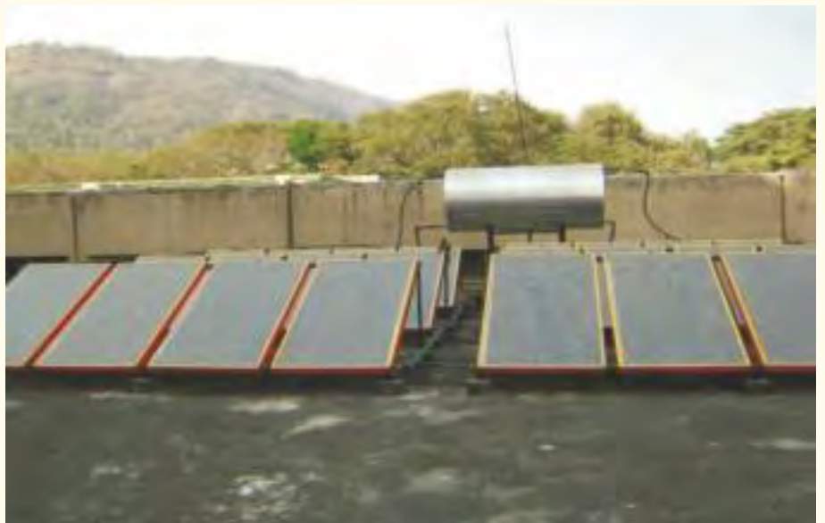
Solar water-heating system
