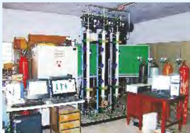
Non-cryogenic helium purification system developed by VECC
