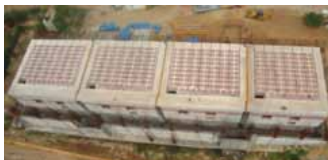
VWSF Phase-I: Thermal Vaults
