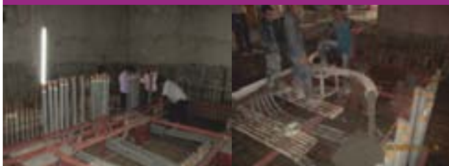
Under floor embedment installation for Hot Cells and Hot Cell area concrete pouring
