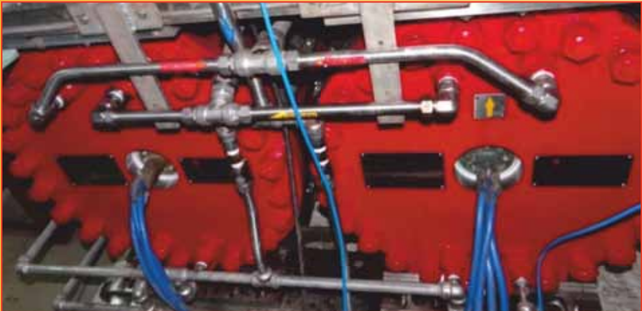
2x25 cell modules at Electrolyser plant
