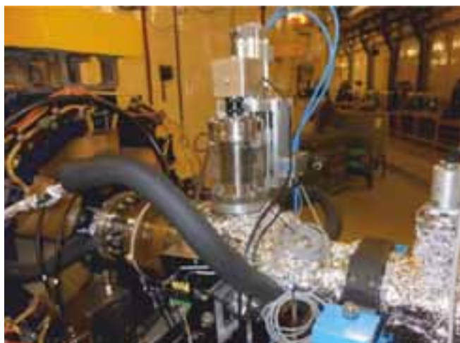
Beam Profile Monitor installed in Indus-2 ring
