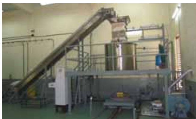
Melt Densification System at CWMF, Kalpakkam
