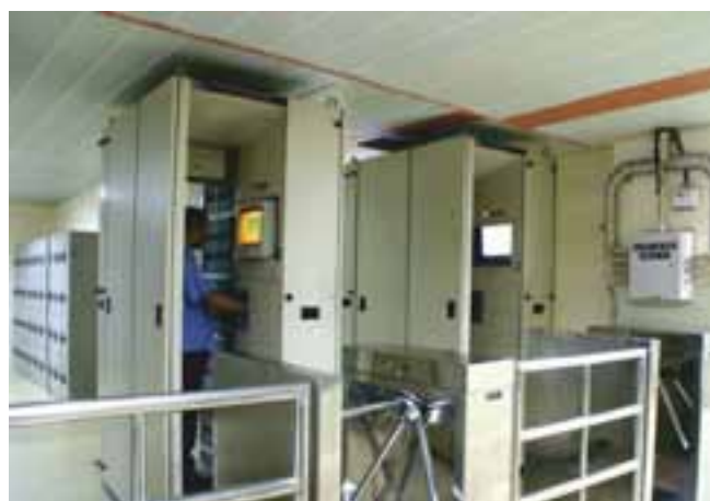
Plastic Scintillator based Portal Monitoring System (PMS)
