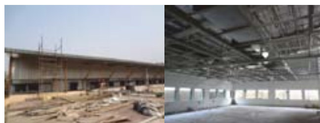
Construction on first floor over RPL extension building (outside view and inside view)
