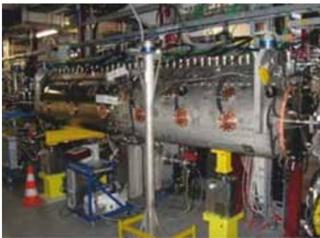
One of the WR 2300 copper coated Stainless steel power couplers installed with the CCDTL accelerating structure of linac-4 tunnel at CERN
