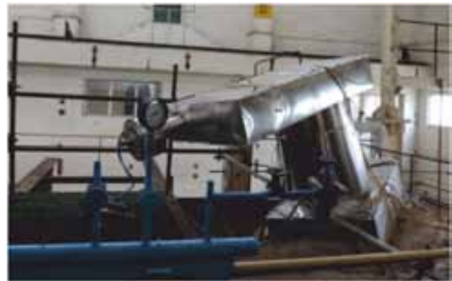
Gate Valve and Shield plug on transfer vessel
