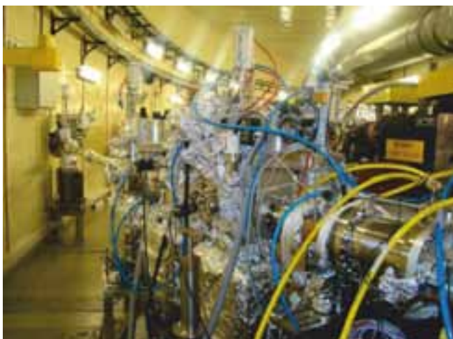
Front end part installed in BL-5 AMOS beamline
