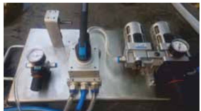
CAROT Control Panel
