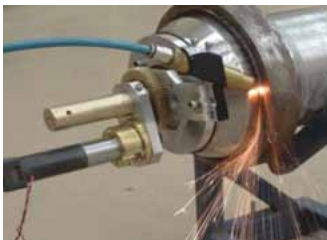
Mock-trial for laser cutting of bellow lip after removal of outboard end-fitting
