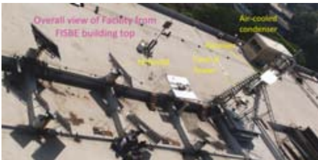
Photograph SOLAR Power TEST Facility while heliostats are focusing on receiver (SOPTEF)
