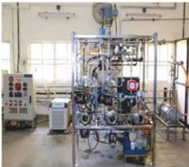
Solvent purification system
