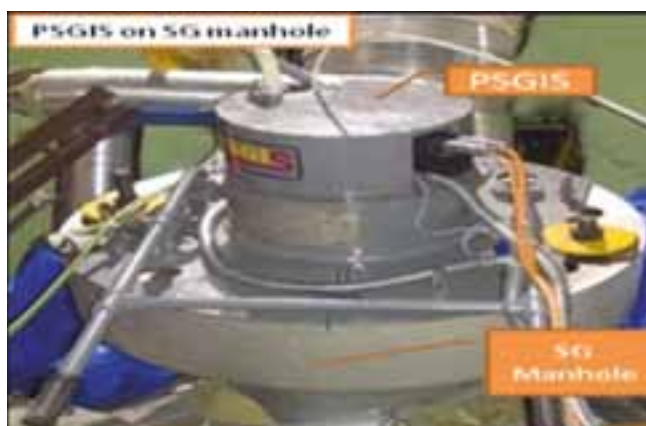
PSGIS device installed on the steam generator
