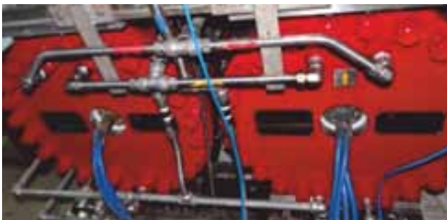
2x25 cell modules at Electrolyser plant
