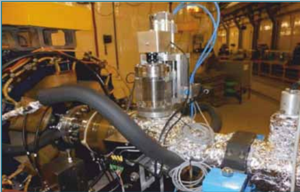
Beam Profile Monitor installed in Indus-2 ring
