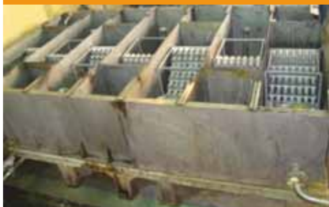
Coalescers placed inside Mixer Settler-2
