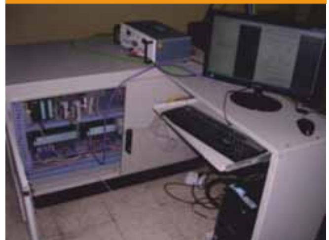
Control System for ADM
