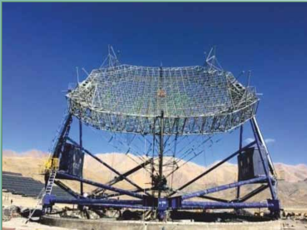
Partially assembled mechanical structure CIMs of MACE telescope as on 30th Nov. 2016
