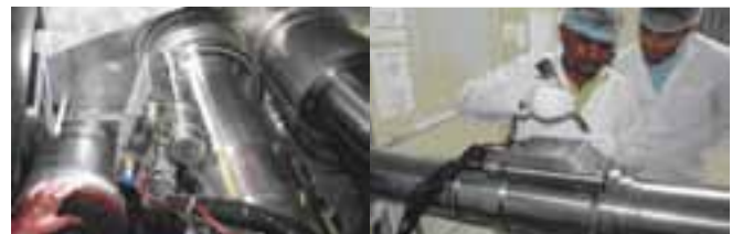
AGMS bellow lip welding in progress and optimizing the AWT parameters at RAPP-7&8
