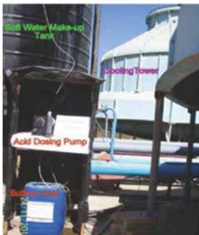
Acid dosing system
