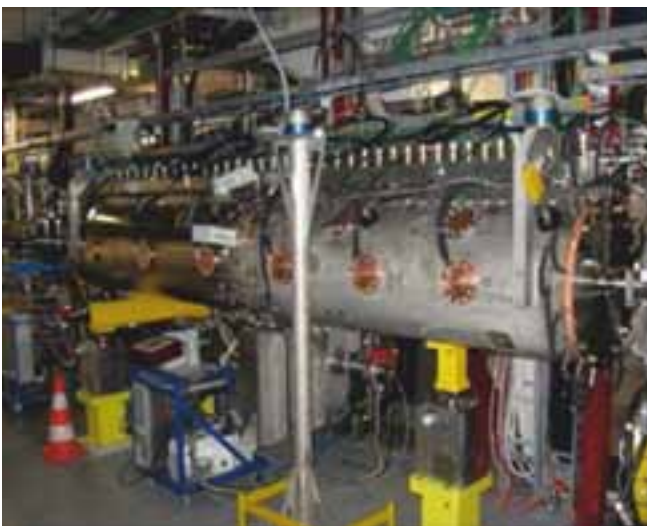
One of the WR 2300 copper coated stainless steel power couplers installed with the CCDTL accelerating structure of linac-4 tunnel at CERN
