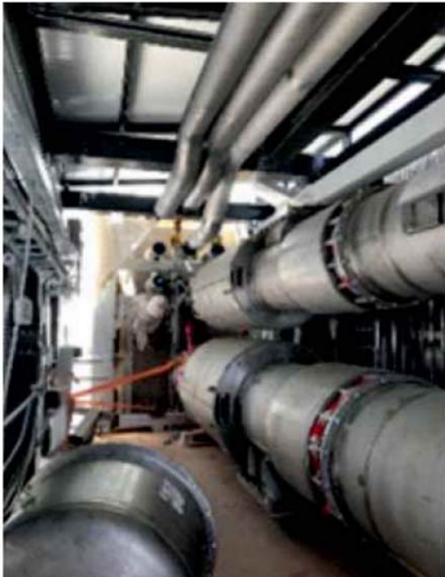
W lines (on top) in cryo-bridge leg connecting B11
