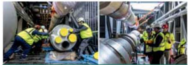
Installation of the seismic decoupling spool being carried out at ITER site
