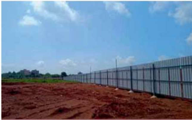
GI sheet fencing at construction area at Homi Bhabha Cancer Hospital in Jatni, Khordha
